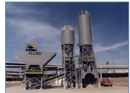
CONCRETE MIX AND LOAD FACILITY
